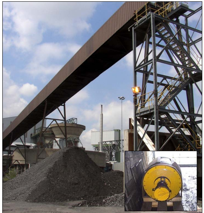
Elevated conveyor discharges tailings at 500 tph. Photo insert shows close-up of 75 kW Rulmeca Motorized Pulley prior to installation.
